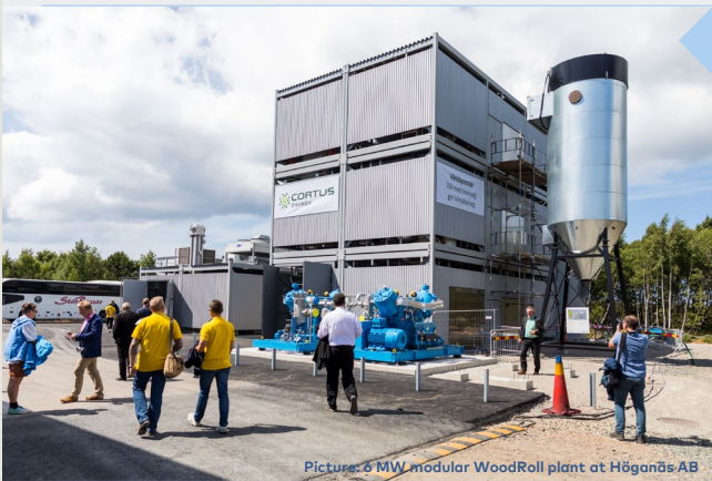
Picture: 6 MW modular WoodRoll plant at Höganäs AB
