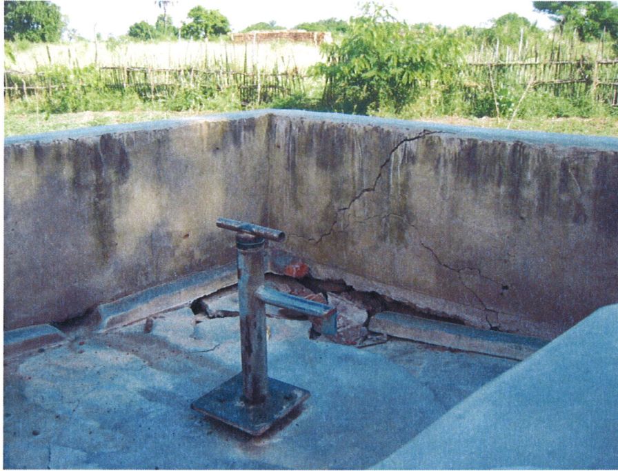
Photo 4: Flood damaged shallow well in Chikadayenda village
