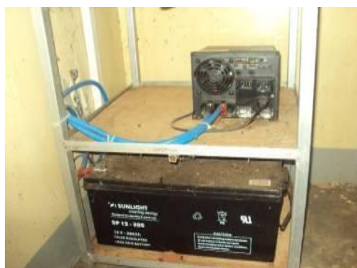
Solar batteries at Bukasa donated by KDDP
